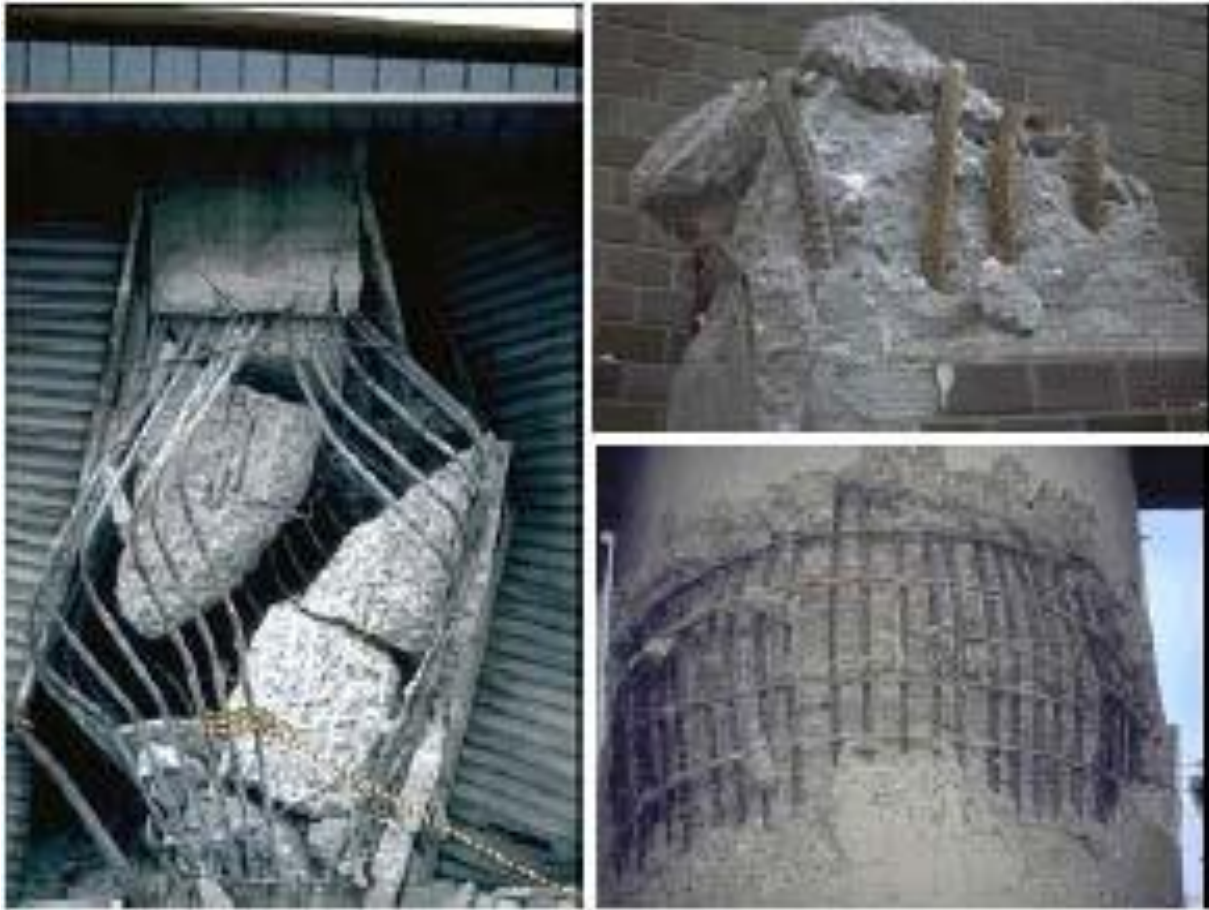
Figure ( 2.6 ): Column failures in Kobe 1995 earthquake
